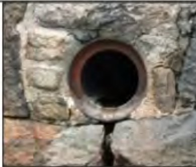
Cracked rock below the outfall may indicate an intermittent discharge.
