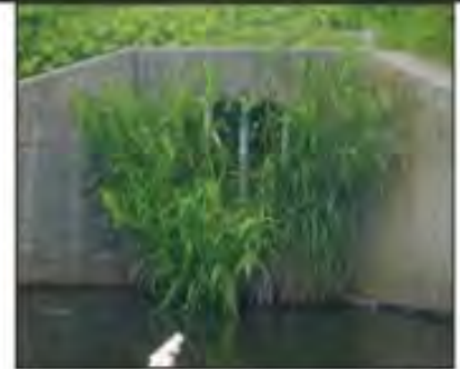
Excessive vegetation may indicate enriched flows associated with sewage.
