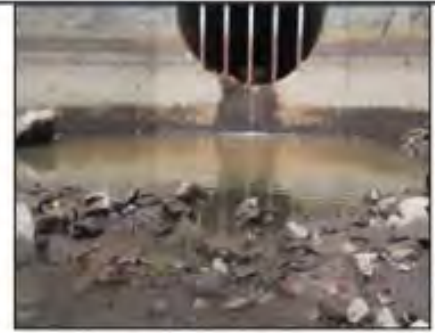
Poor pool quality. Consider sampling from the pool to determine origin.
