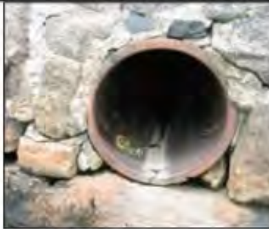
Staining at the base of the outfall may indicate a persistent, intermittent discharge.
