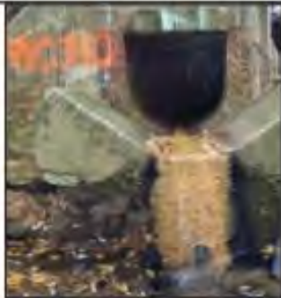
Brownish stain of unclear origin. May be from degradation of the brick infrastructure.
