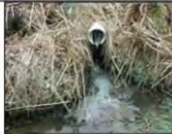
Failing Septic System: Turbidity Severity: 3
