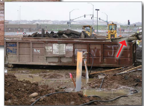
Figure 2. Chute washwater leaking from a roll-off bin being used as a washout container
